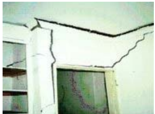
Figure 2. Failure of super-structure.
