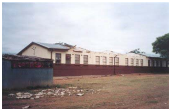
Figure 4. Portion of a roof blow away.
