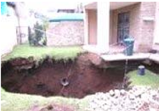
Figure 1. Sinkhole formation on dolomites.
